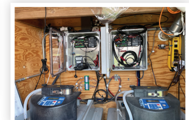
USGS equipment inside the new Phosphorus Removal System (PRS) gage house will look similar to the inside of the current Bioreactor gage house. The equipment enables remote monitoring and sampling to occur before and after the PRS, while also providing real time data to the public. Photo Credit: Joe VanHulle, Natural Resources Conservation Service (NRCS)
