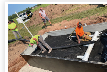
Constructing the inlet manifold and distribution tile system on top of geotextile in the concrete holding tank. Below the geotextile is 8" of activated alumina, followed by another layer of geotextile, and the outlet manifold and distribution tile system bedded in clean stone. Photo Credit: Joe VanHulle, Natural Resources Conservation Service (NRCS)
